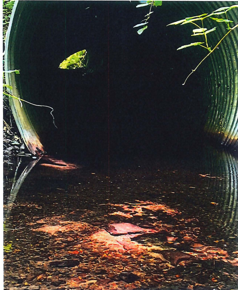
A large culvert in Hubbard Creek shows signs of instability, with both bend and a broken section in the center of the road fill. Failing culverts like this present a significant risk to source water quality.
