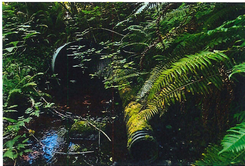
Culvert on the access road from Vista Drive showing odd drainage structures and partially failed primary culvert in Hubbard Creek.
